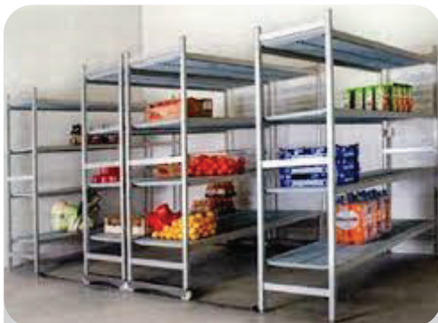
Chiller & Freezer Room
