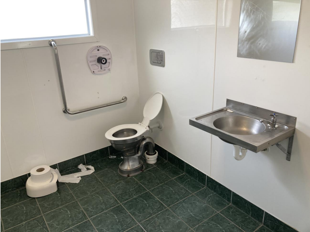
Figure S3-2: Example of a toilet with a broken toilet paper dispenser (photograph by first author, 2021)
