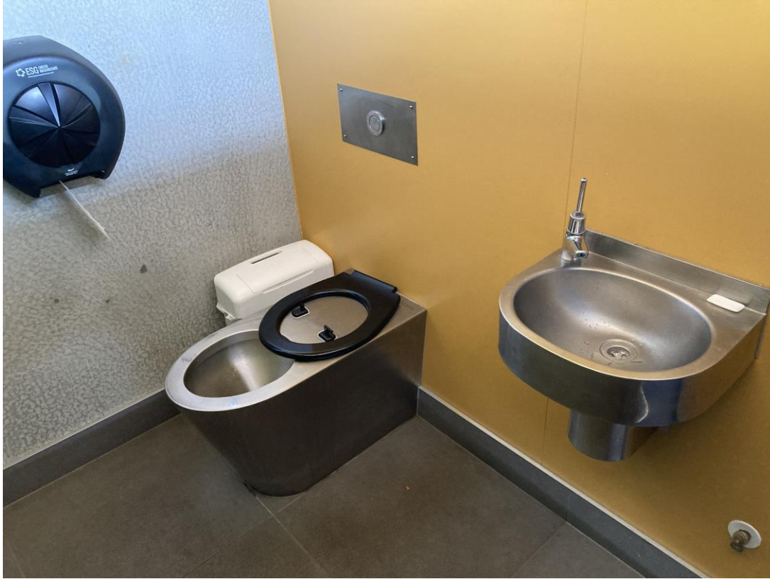
Figure S3-1: Example of a broken toilet seat which also has no lid. This photo also shows a lever for activating the tap and a cake of soap (photograph by first author, 2021)
