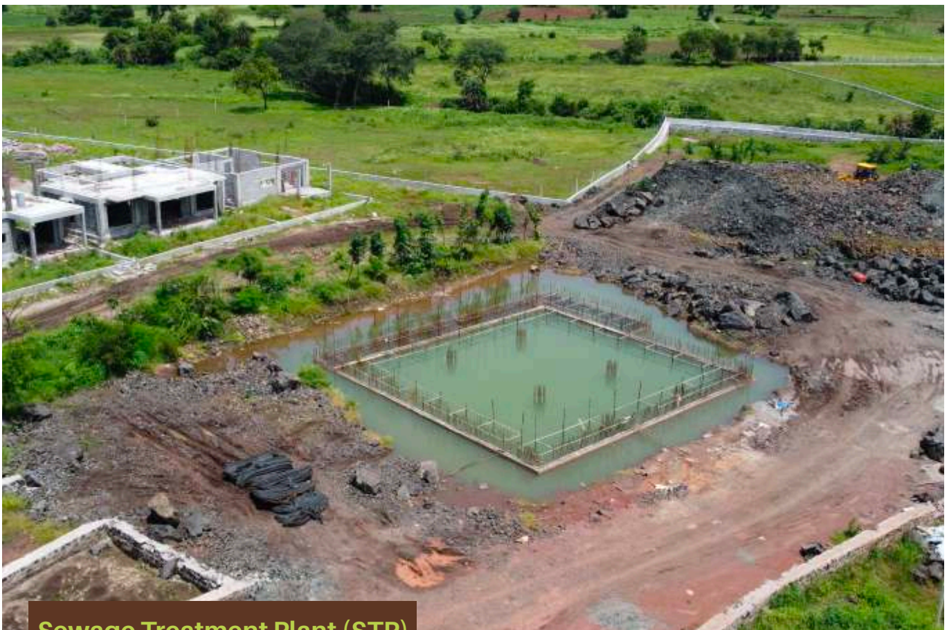
Sewage Treatment Plant (STP)
