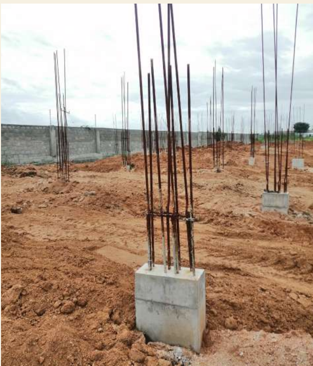
Soil filling up at the pedestal level has been completed for the North facing villas
