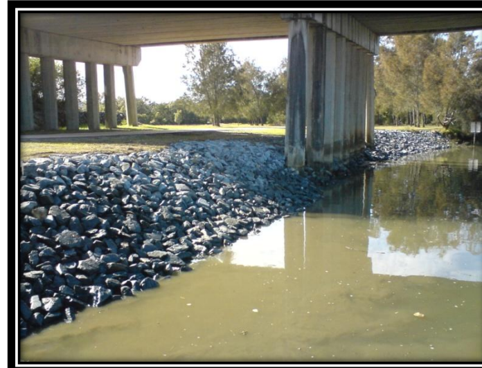
Saltwater Creek - after bank stabilisation by Gold Coast Barges with rock armouring.
