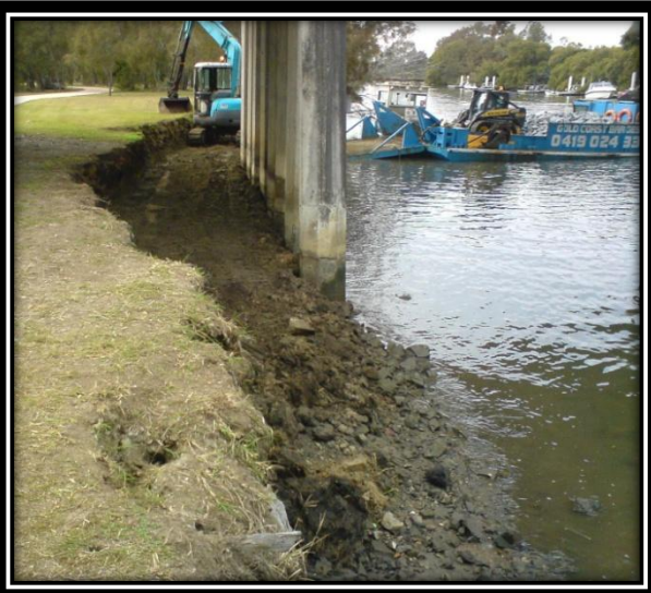
Saltwater Creek before Gold Coast Barges was engaged by GCCC to correct bank erosion issues.
