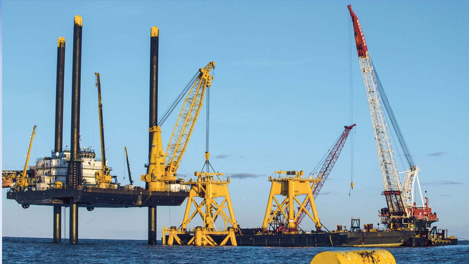
L/B Robert (MiNO 335 Class) installed piles and topsides for the Block Island Project
