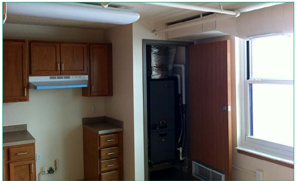
Figure 1. Orness Plaza, a public housing complex in Mankato, Minnesota. Between 2010 and 2012, the property was renovated to meet Enterprise Green Communities criteria and LEED® Silver certification. The photos document HVAC improvements that were part of the renovations, including range hoods that vent outdoors. The project was part of a US Department of Housing and Urban Development (HUD)-funded research project that the National Center for Healthy Housing (NCHH) conducted. Photo courtesy Blumenthals/Architecture.
