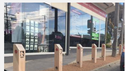
Timber Bollard: Access restriction, unknown containment, impact behaviour unknown- deemed frangible in one direction.
