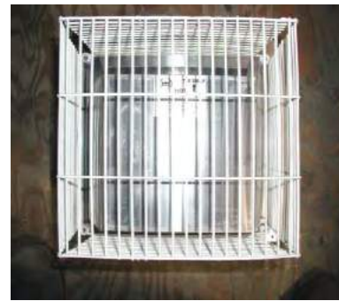
VIEW OF SAFETY CAGE
