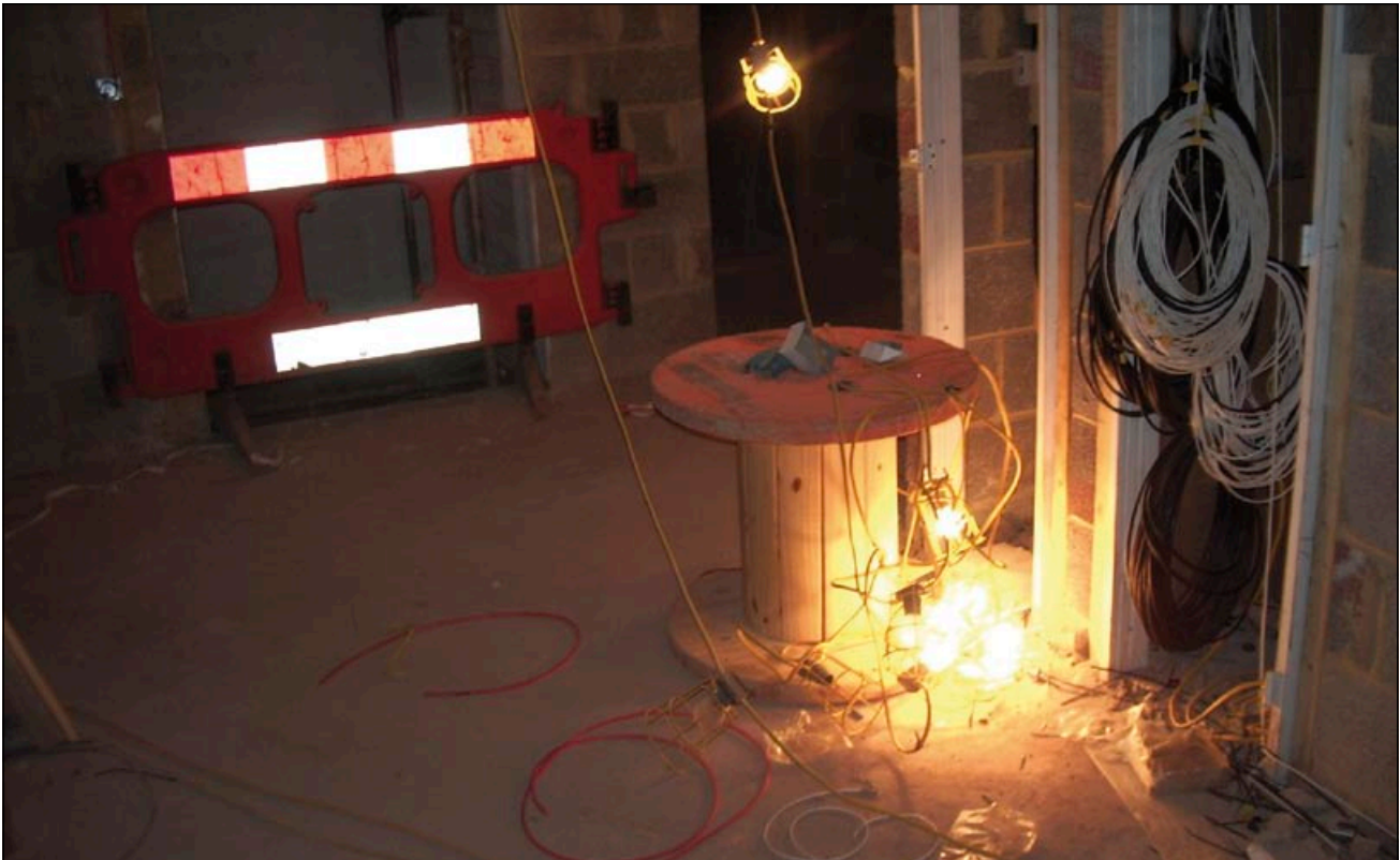
Figure 2 Festoon lighting: an incorrect fixing creates a potential fire risk
