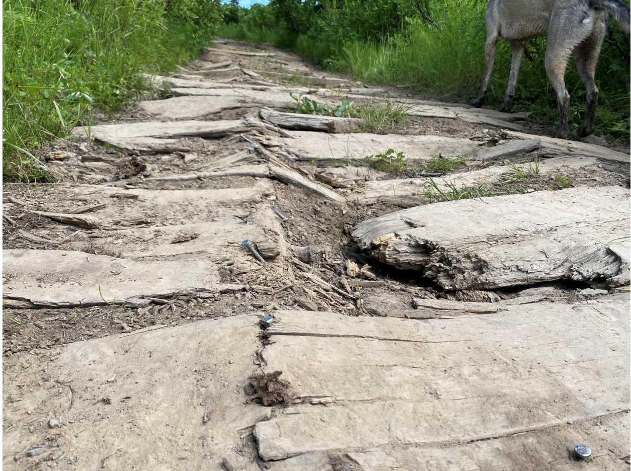
Photo 1: A close-up of the degraded Boardwalk Trail that users avoid. Big nails are sticking up everywhere, which stops both horse riders as well as ATV users. July 2022.
