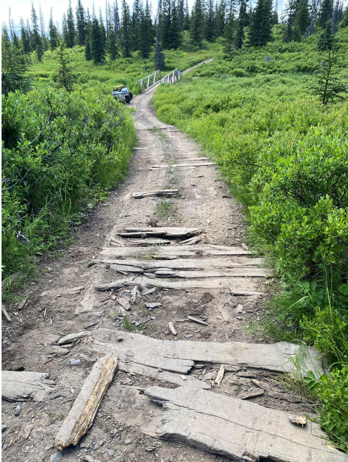
Photo 2: Moose Creek bridge on Boardwalk Trail looking west from the beginning of the 1.4 mile severely degraded section that is shown in photo 1.
