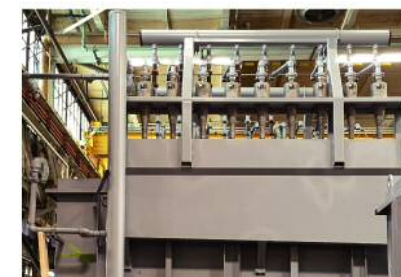
Large flow rate filtration for centralized tank
