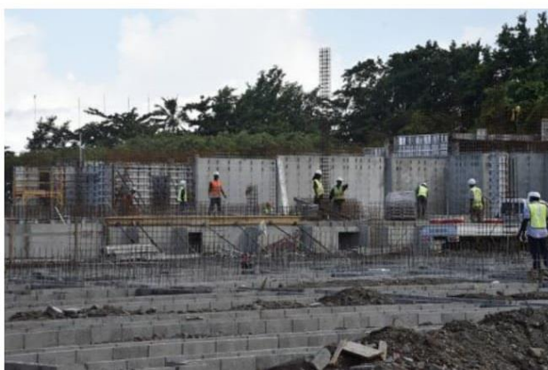
Construction in progress by Range Development at the Cabrits Resort Kempinski at Douglas Bay in Portsmouth
