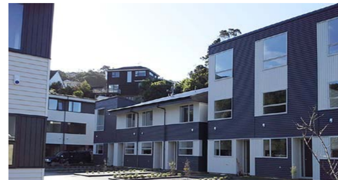
Elevate Apartments All External walls and finishes, carpentry trade for apartment building in Taranaki Street, Wellington. Client: T-Street Holdings Ltd. Architect: Architecture+ Engineer: Aurecon Value: $3.2m
