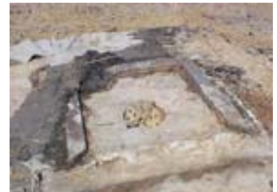
Photo 3: Redwood strips surrounding inlet/outlet structure at bottom of a pond.
