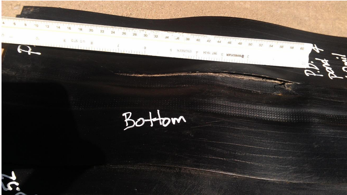
Figure 1: Geomembrane defect below intact dual-track geomembrane seam under the salvage edge of the geomembrane. The Air Lance test is able to detect such defects located outside of the dual-track geomembrane seam even though the air channel passes the required pressure test according to ASTM D5820 or D7177.
