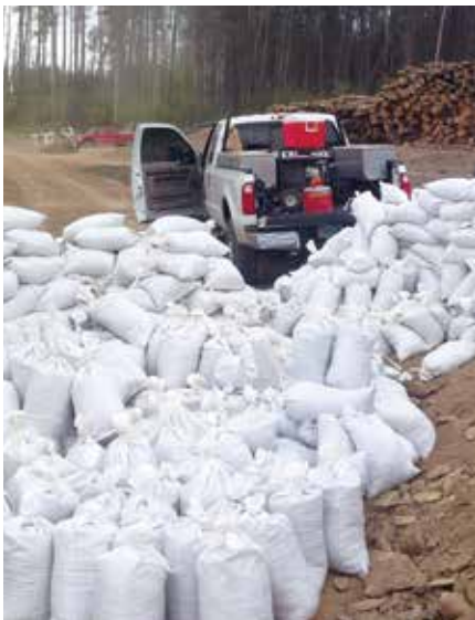
More than 1,000 sandbags were used to hold geomembrane panels in place before welding.
