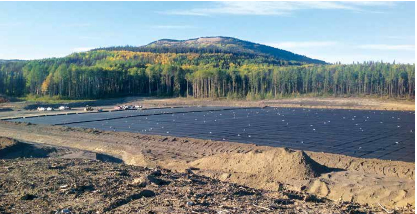
For the Tumbler Ridge project, more than 780,000 SF of geomembrane was pre-fabricated; and installed in eight days.
